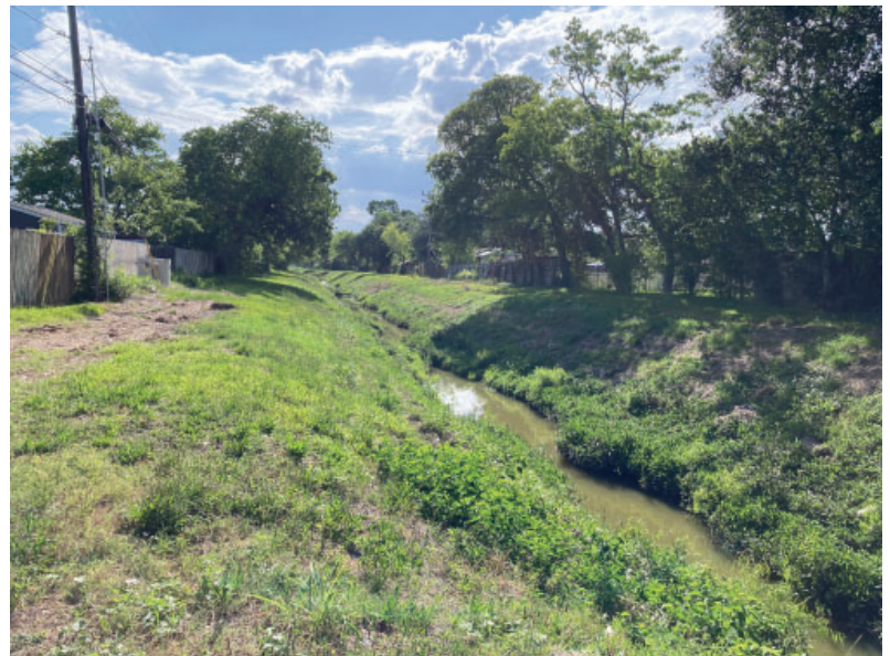
Figure 39: View of open drainage ditch in close proximity to single family residential homes.
