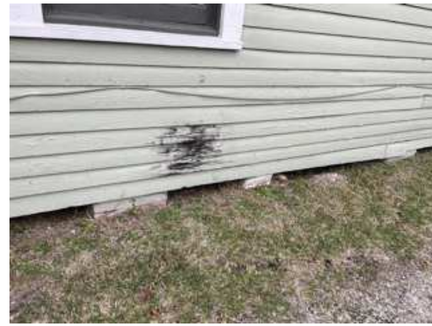
IMAGE INDICATES PORTION OF WALL WHERE SIDING HAD BEEN DETERIORATING, TO BE REPLACED WITH SIMILAR NEW SIDING
