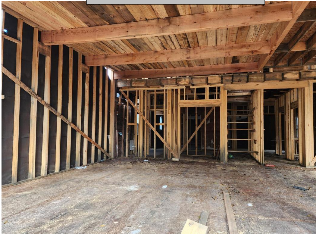
Right Rear Elevation. Window Openings Removed
