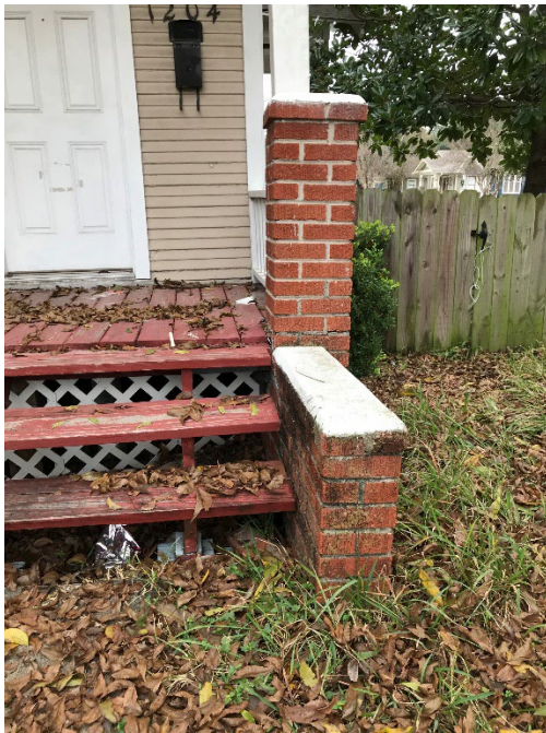
Figure 12 - Leaning brick stoops with gapped mortar joints
