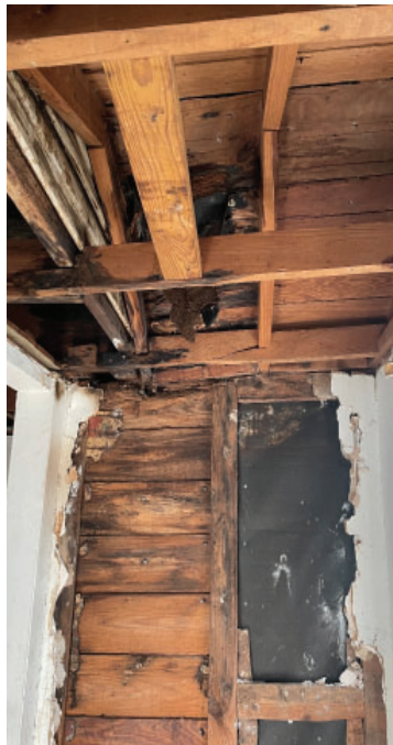
Existing Structural Damage at Garage Structure
