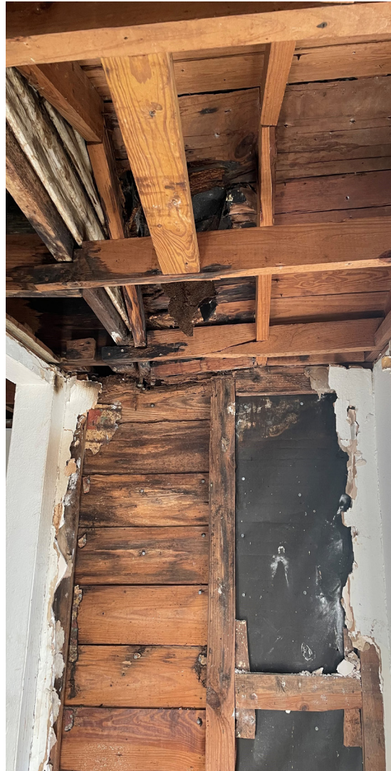
Existing Structural Damage at Garage Structure
