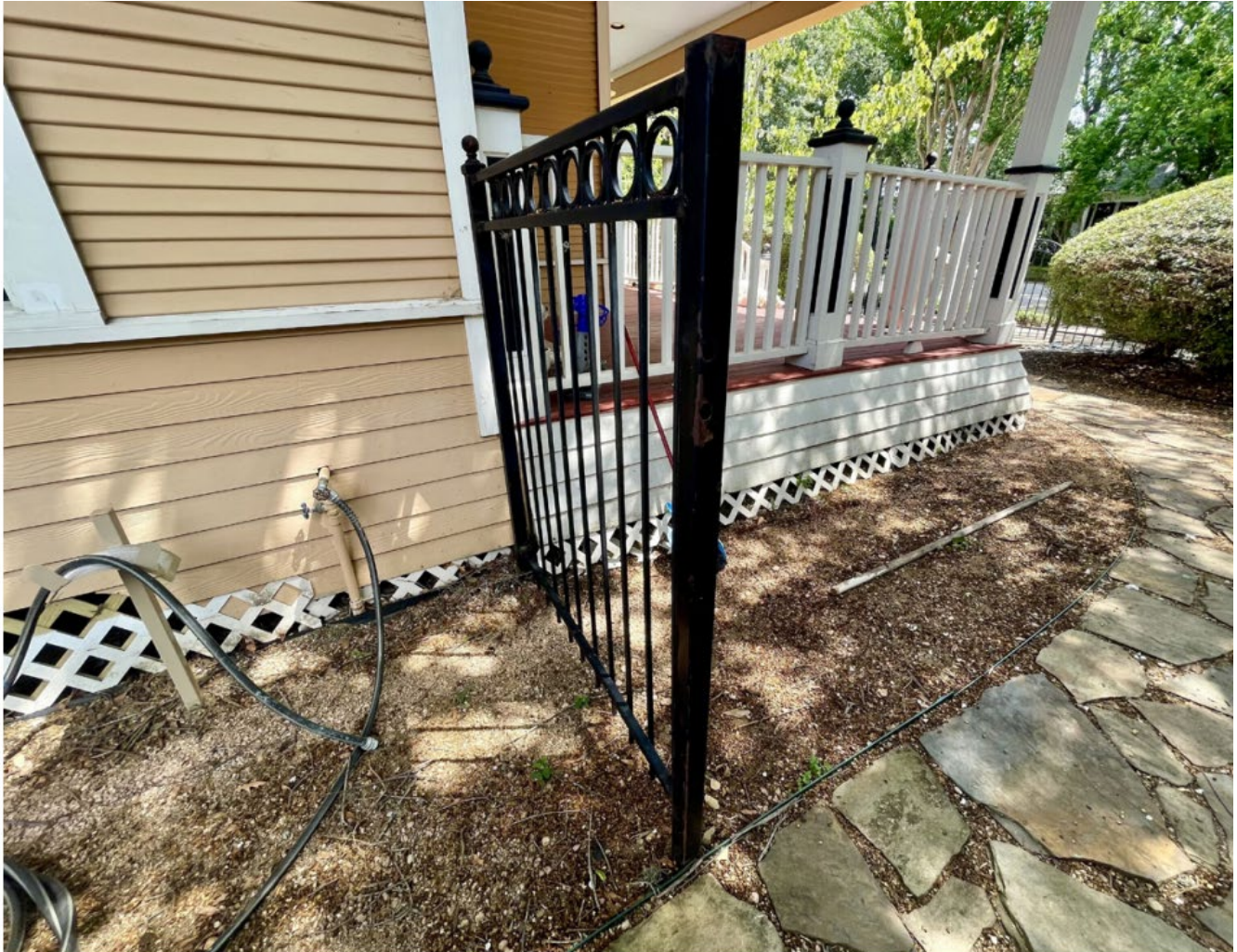
Siding on South Side (Skirt and siding below window water table to be revised)
