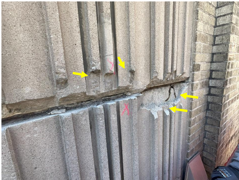
Photo No. 2. View of spalled cast stone unit with exposed reinforcing steel.
