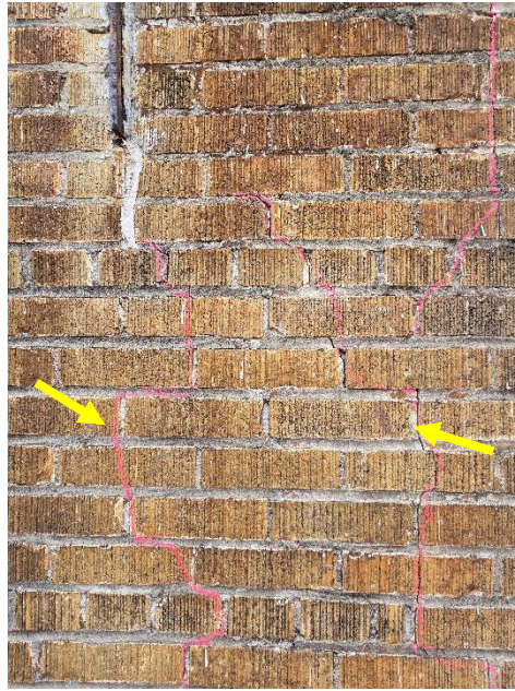
Photo No. 7. View of step cracks in brick masonry designated to be sealed. The cracking appears to stem from the embedded steel near the upper left corner of the image.
