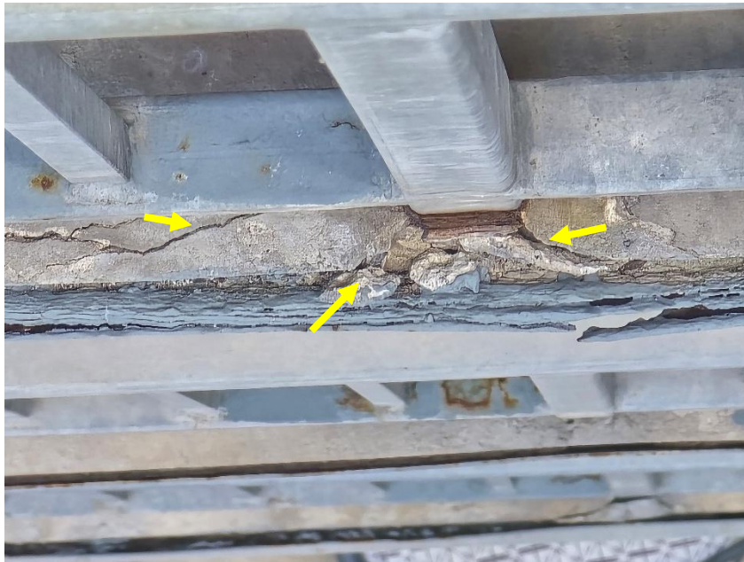
Photo No. 10. View looking down at the cracked and spalled concrete near a balcony post embed. The perimeter steel angle is also corroded.
