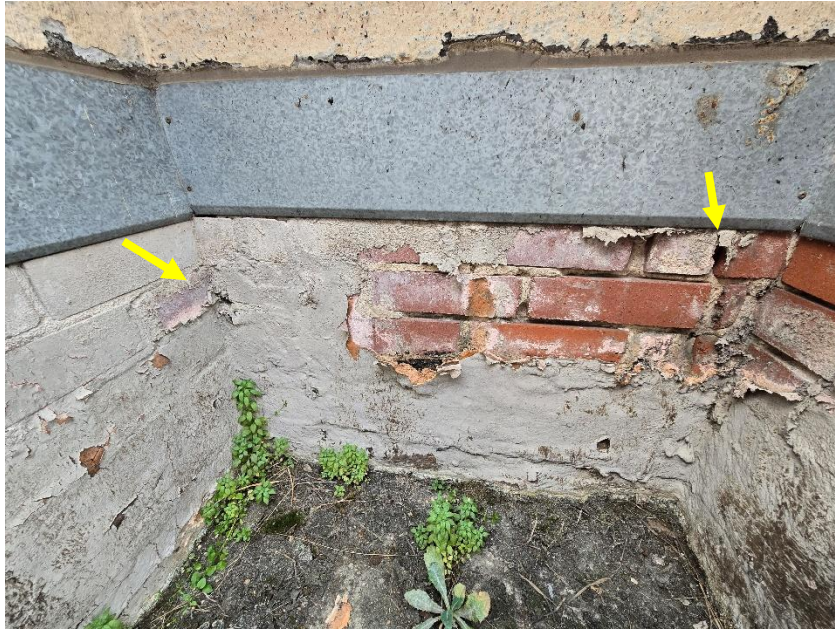
Photo No. 5. View of inboard side of the masonry parapet with eroded mortar joints and peeling coating.
