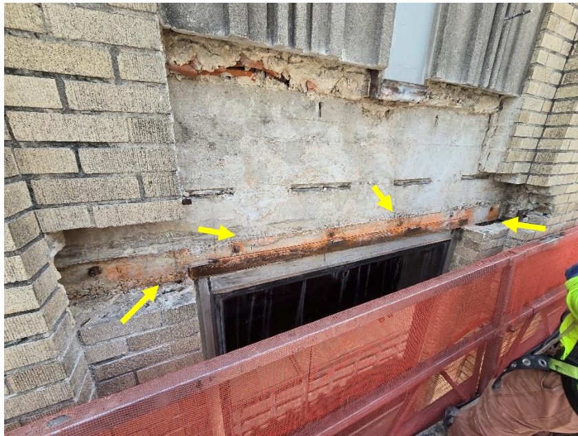
Photo No. 4. View of removed shelf angle at cast stone spandrel with cut anchors and exposed secondary angle at the window head.
