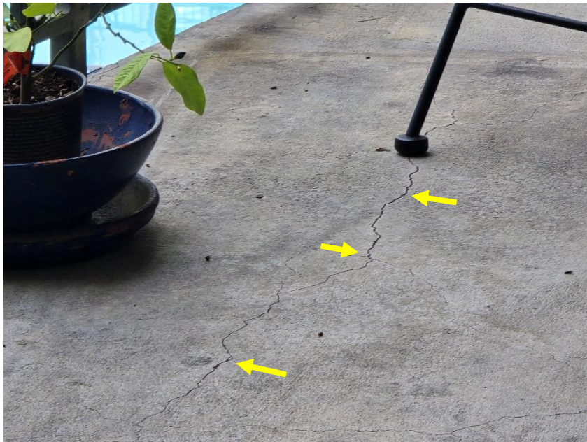
Photo No. 12. View of concrete balcony slab crack.
