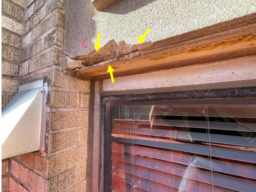
Photo No. 1. View of spalled cast stone spandrel units.
