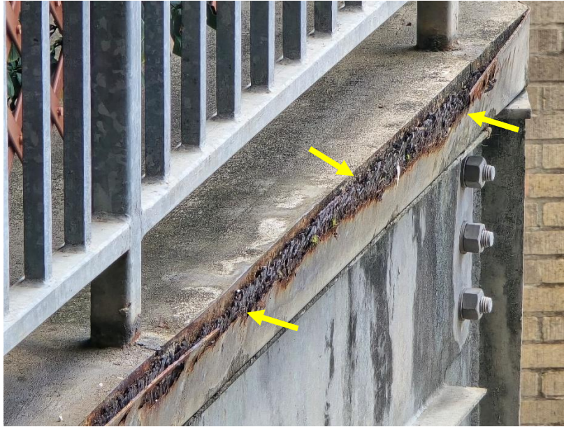
Photo No. 11. View of corroded steel angle at balcony slab edge. Moisture is likely getting trapped between the concrete and the steel.
