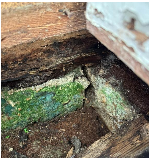
Photo 11 – Cracked grade beam and rotting sill
