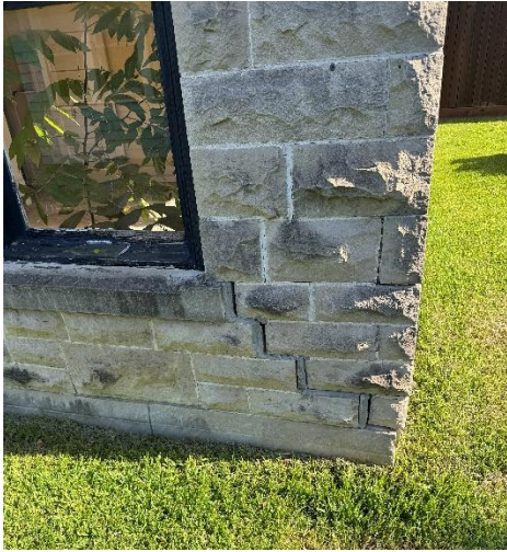
Photo 7 – Veneer cracks at SE corner
