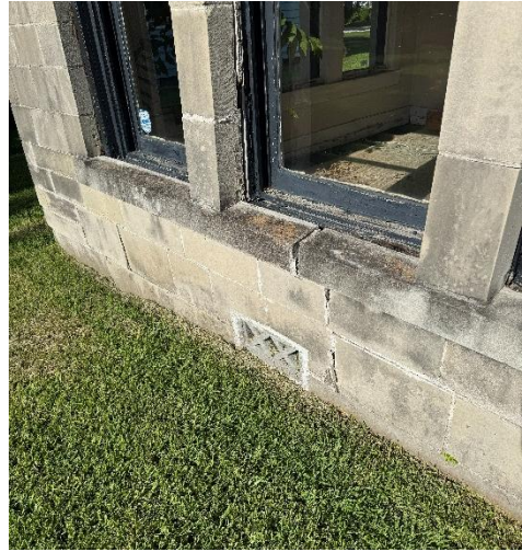
Photo 8 – Veneer cracks at east elevation
