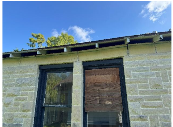
Photo 10 – Veneer cracks at south elevation
