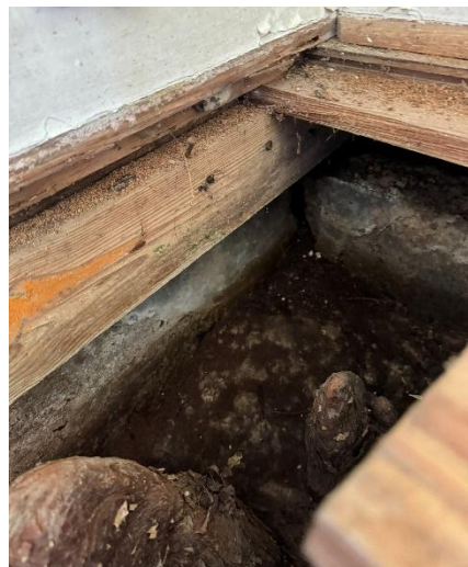
Photo 12 – Cracked grade beam and rotting sill
