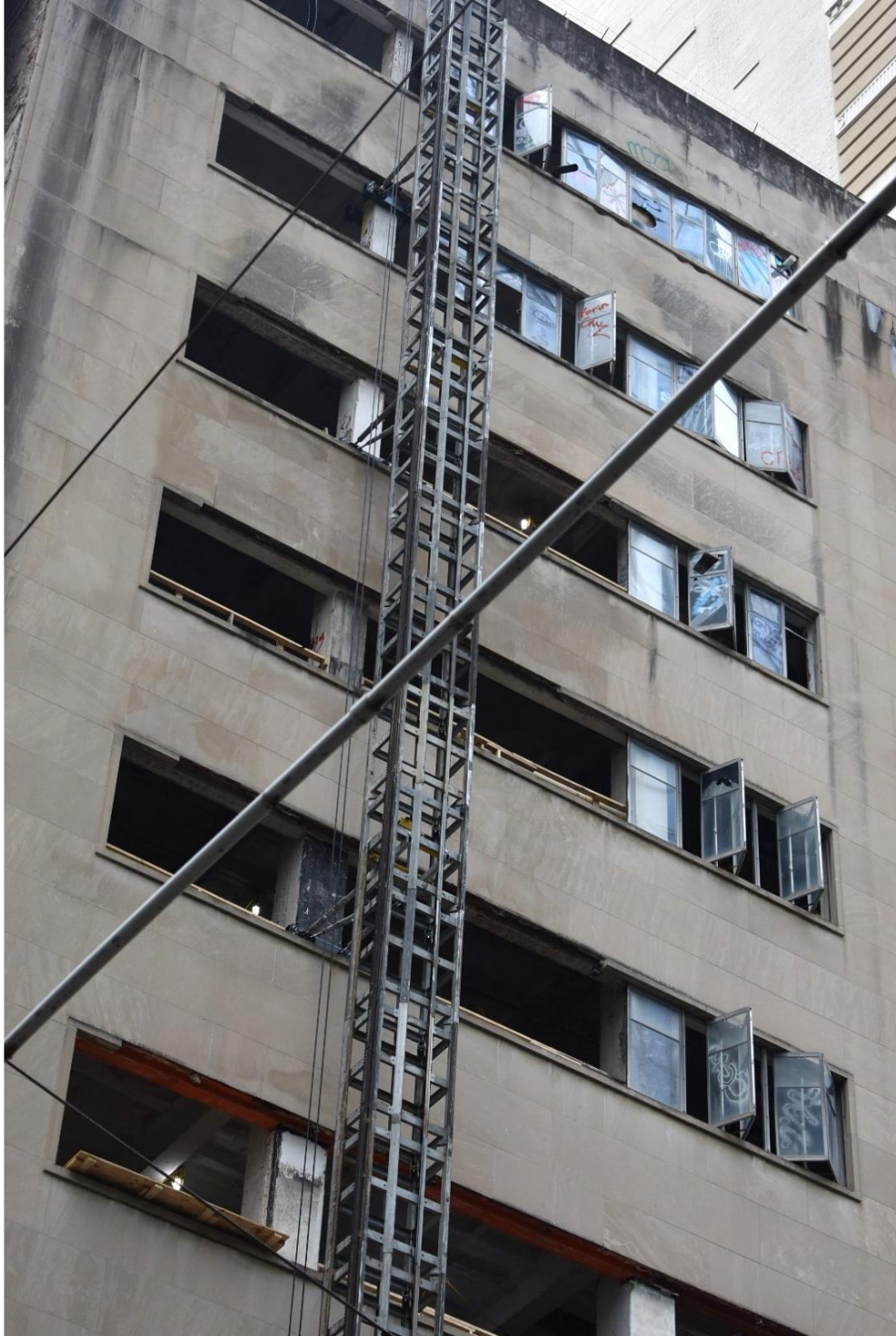
Photo 6: East elevation facing Main Street, detail of upper floors ribbon windows; view north.
