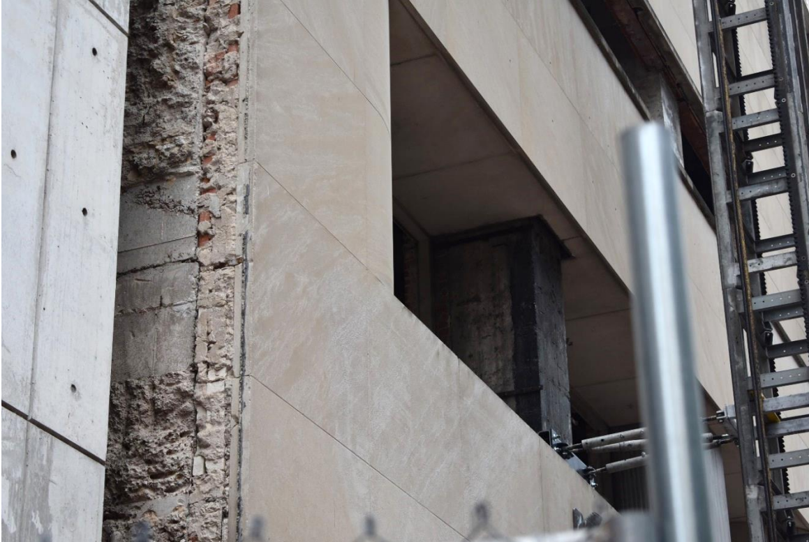
Photo 15: East elevation facing Main Street, fourth floor and south elevation exterior; three-quarter view north.
