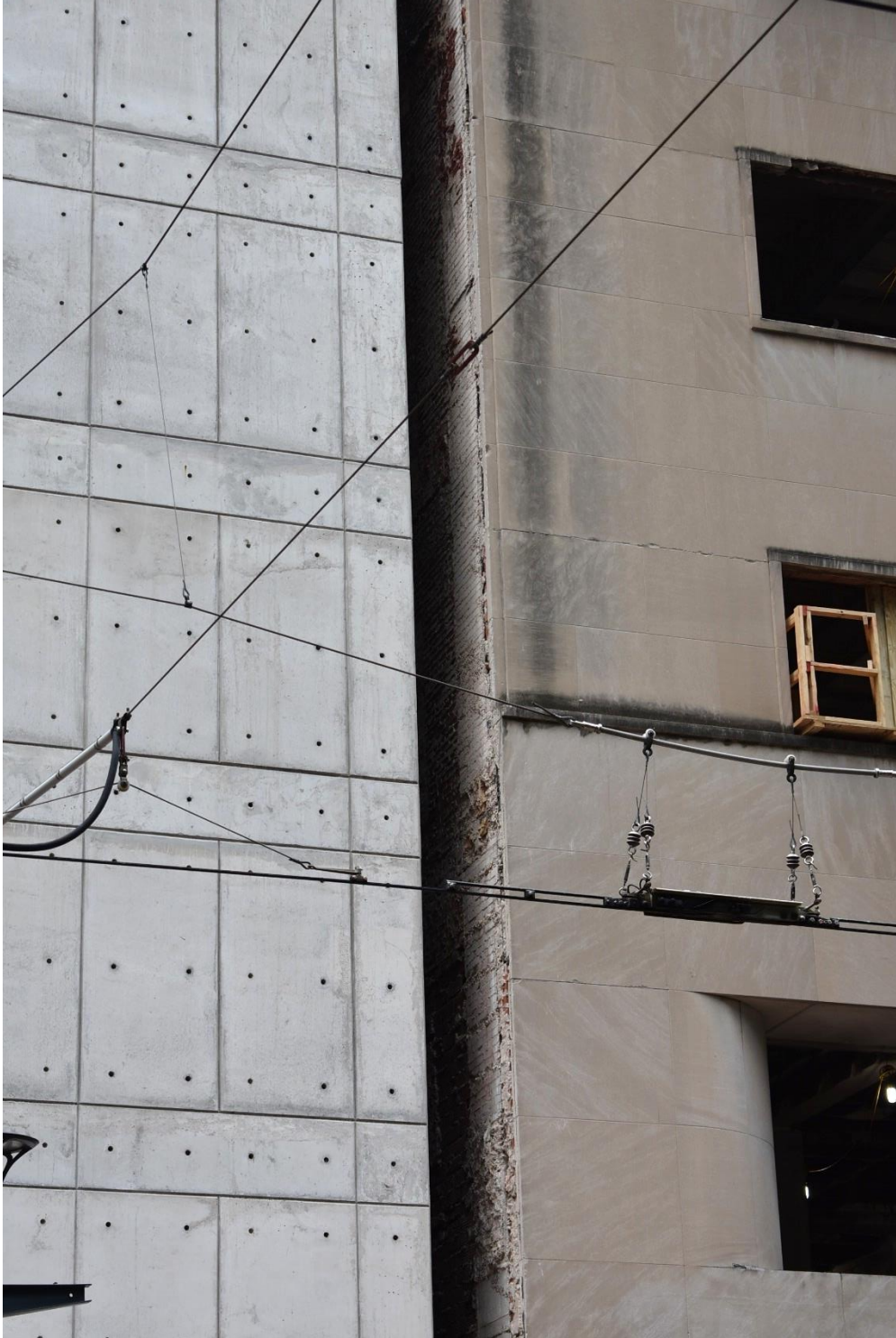
Photo 8: East elevation facing Main Street, detail view of exterior limestone and brick; view north.
