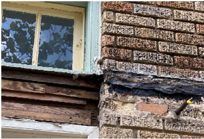
Photo 7 – No visible flashing at removed awning connection
