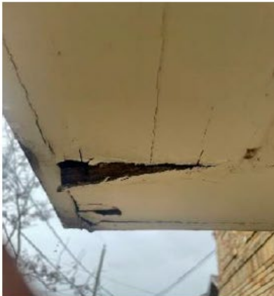
Photo 3 – Soffit damage at awning
