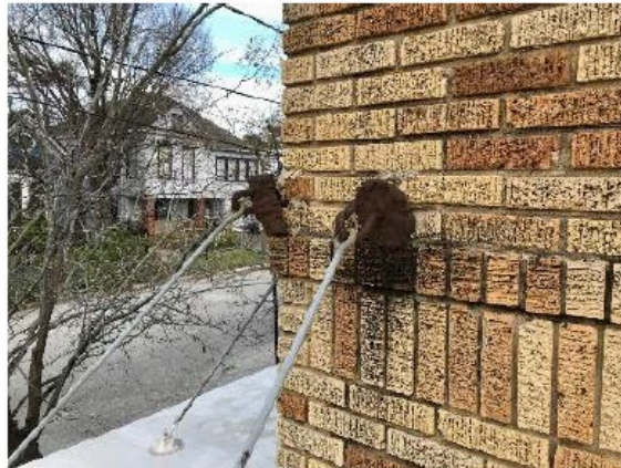
Photo 4 – Failing connections at existing awning
