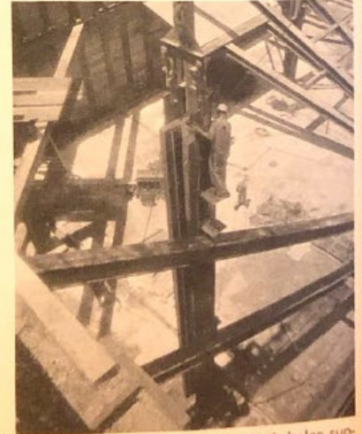
Workmen place a column which helps support framing for the first two basement floors below ground level.
