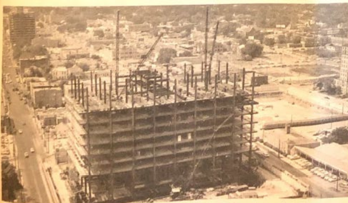
Steel erection has reached a height of 10 floors at this point and decking is being placed on the eighth floor.
