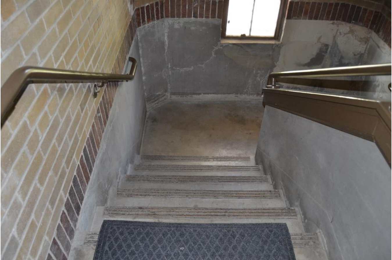
Photo 13. Interior stairwell within the stairwell ell on the side southwest façade. Camera facing southwest.
