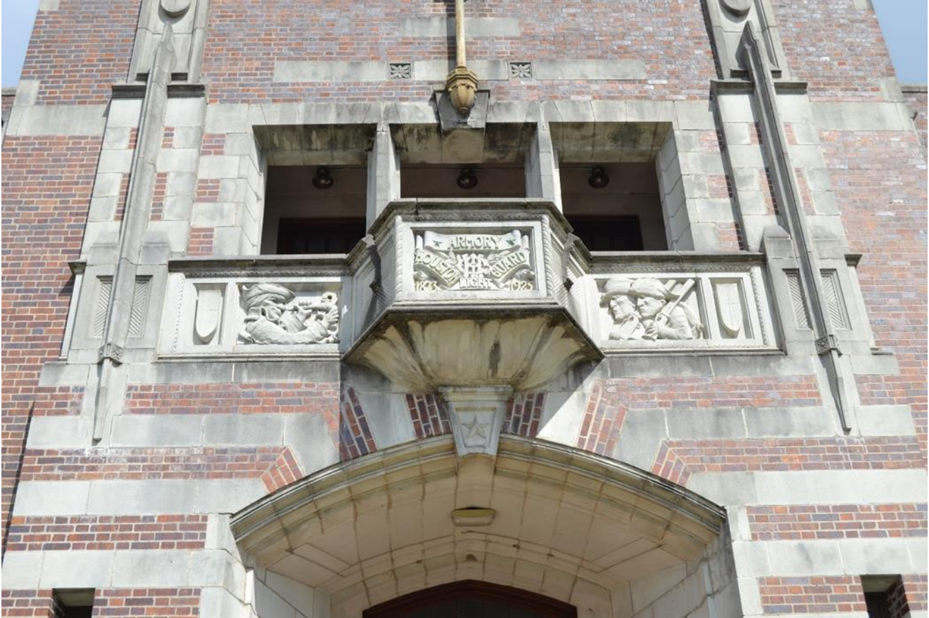
Photo 8. The inset balcony above the historic primary entrance on the southeast façade. Camera facing northwest.
