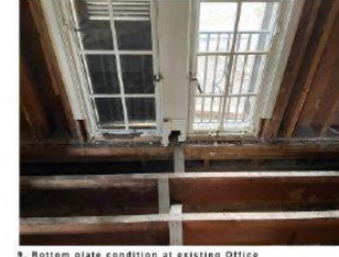
9. Bottom plate condition at existing Office
