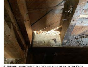
8. Bottom plate condition at east side of existing Entry
