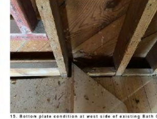
15. Bottom plate condition at west side of existing Bath 02
