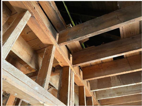
Joists are currently pulling away from structure as wall opposite continues to pull away from existing structure.
