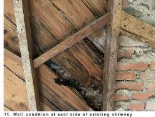
11. Wall condition at east side of existing chimney
