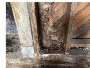
5. Bottom plate condition at west side of existing fireplace
