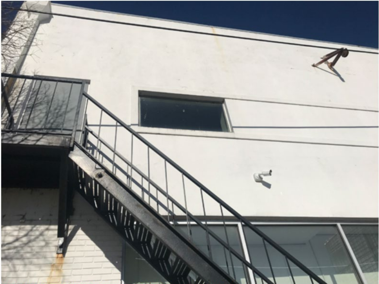
East Elevation Detail, fixed windows at second level and fixed in place historic emergency stair
