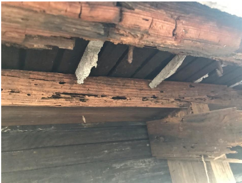
Figure 7-View in porch wall cavity showing water rot of original framing members
