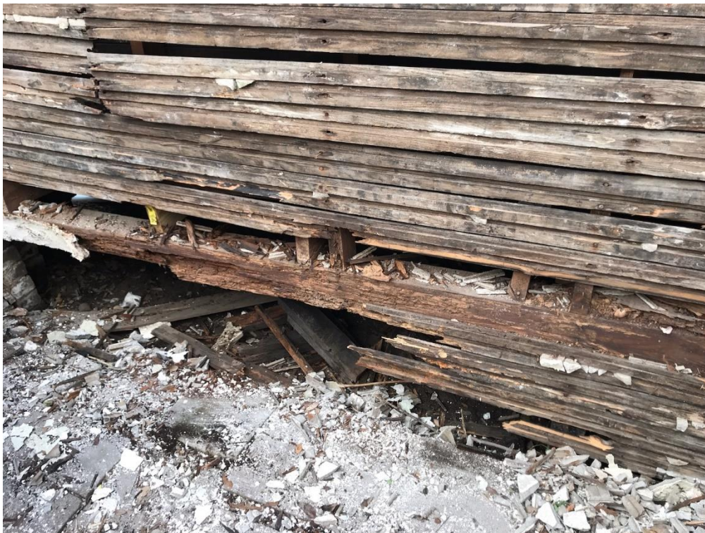
Figure 9 - Image of lower portion of East wall indicating perimeter beam damage.
