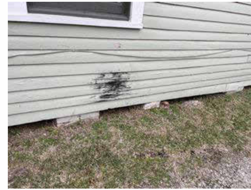
IMAGE INDICATES PORTION OF WALL WHERE SIDING HAD BEEN DETERIORATING, TO BE REPLACED WITH SIMILAR NEW SIDING
