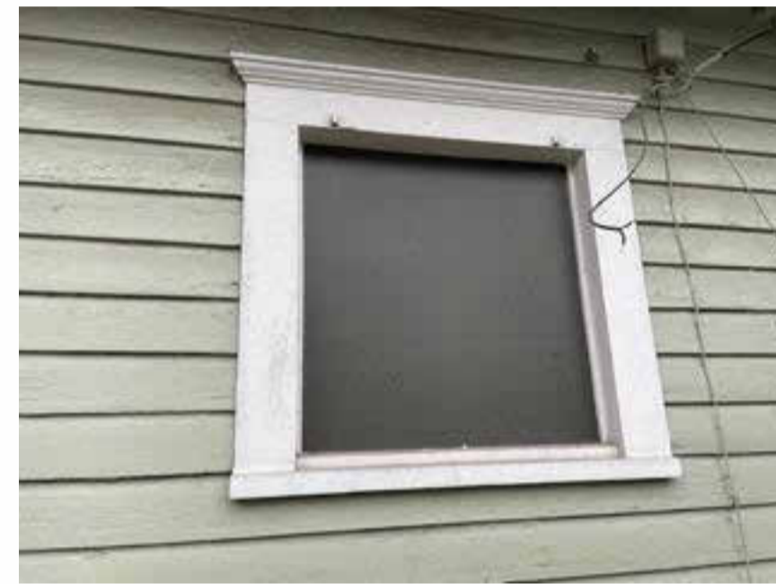
IMAGE INDICATES ORIGINAL WOOD SASH REPLACED WITH PAINTED PLYWOOD PANEL
