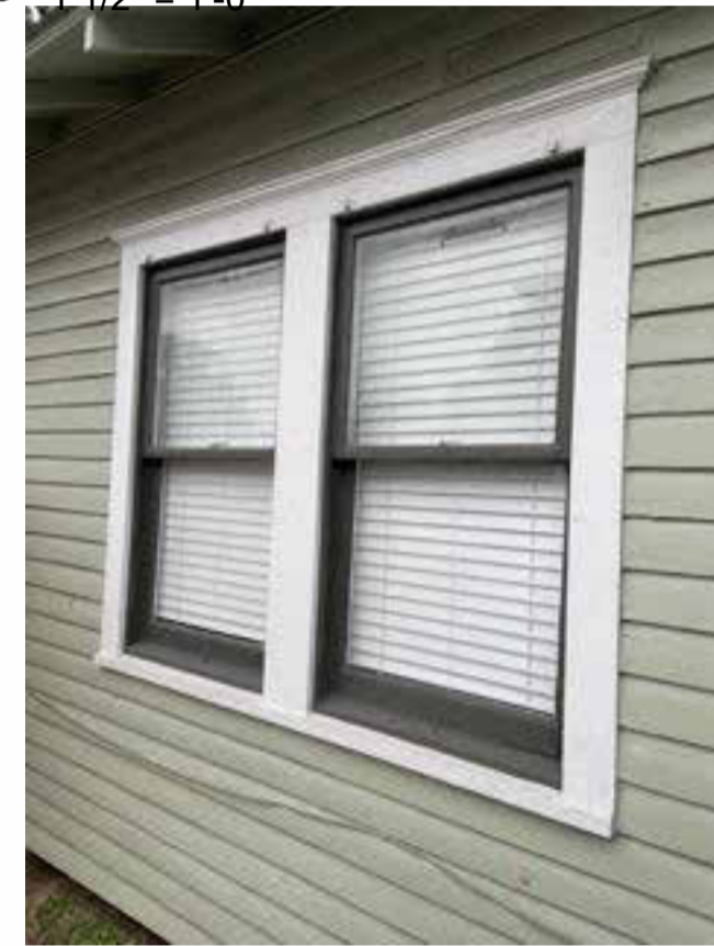
IMAGE INDICATES STYLE AND CONDITION OF THE MAJORITY OF THE EXISTING WINDOWS
