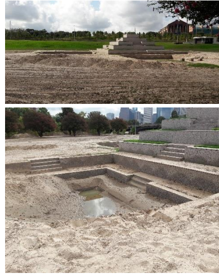
Houston Police Officer's Memorial Artist: Jesus Moroles/ FountainWorks + Veazey HPARD Buffalo Bayou Park District C In Progress Budget: $30,000 Reaffixing loose granite sections. Fountain repair after each Buffalo Bayou flood.
