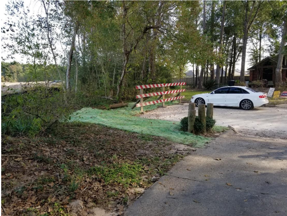
Curlex Blanket Stabilization on Village Springs Drive Note: Light sediment at dead end
