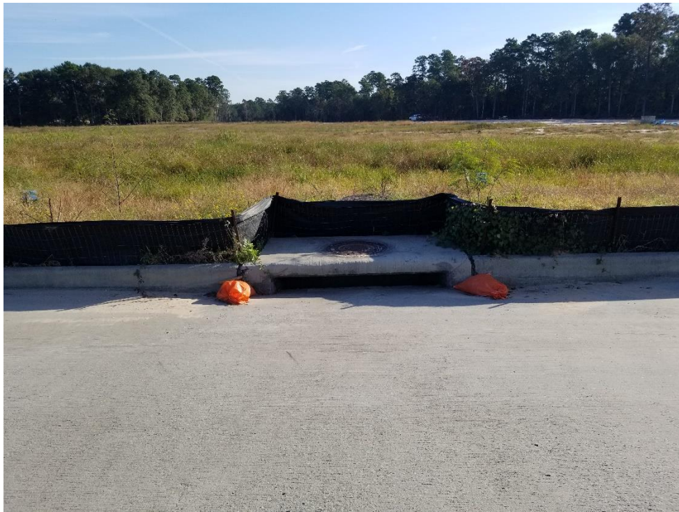
Inlet Protection on Woodland Hills Drive Note: Small amount of silt accumulation
