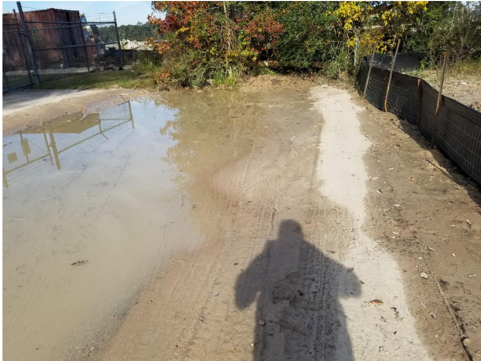
Fair Grove Driveway Near COH Well #6 Note: Ponding and sediment accumulation
