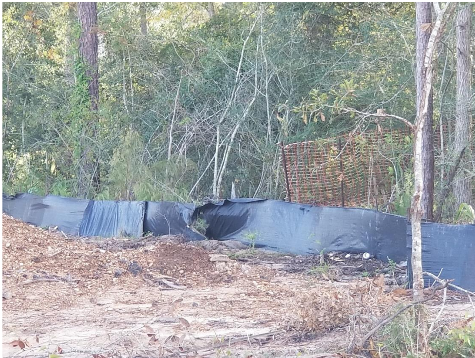
Hole in Silt Fencing Near Fair Grove Drive
