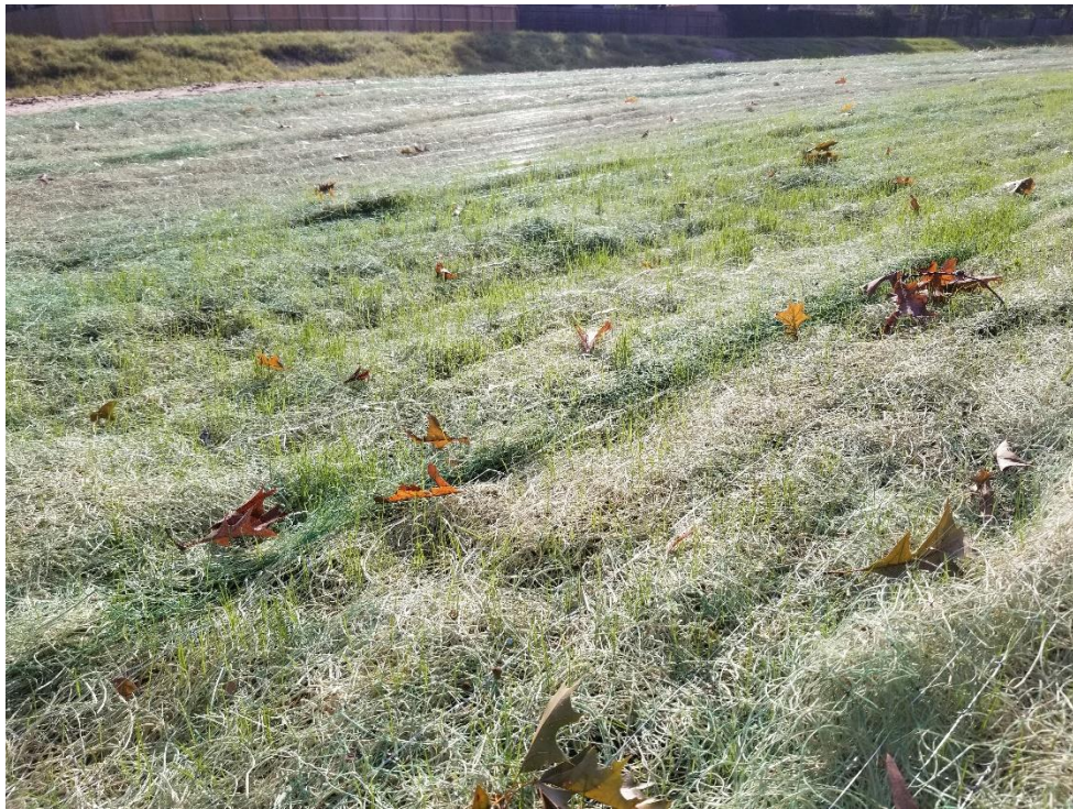
Close View of Curlex Blanket at Creek Manor Drive Note: Grass is beginning to sprout
