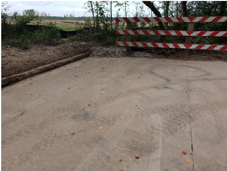
End of Village Springs Drive Note: Thick sediment has been removed
