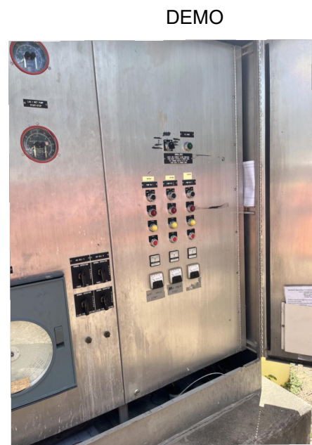
EXISTING LIFT STATION CONTROL PANEL NTS
