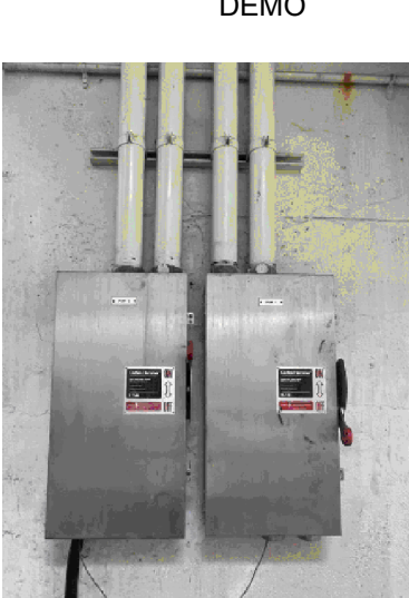
EXISTING PUMP MOTOR DISCONNECT SWITCHES
