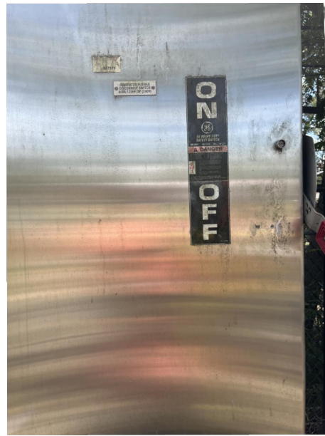
EXISTING LIFT STATION MAIN DISCONNECT NTS
