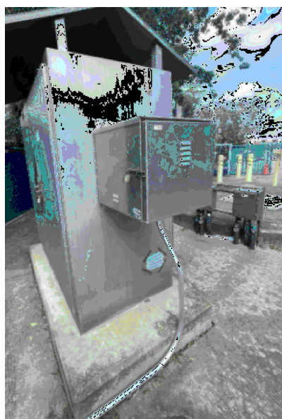
EXISTING WIMAX CONTROL BOX NTS
