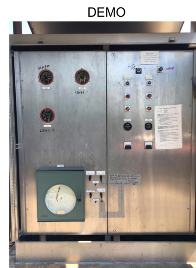
EXISTING LIFT STATION CONTROL PANEL
