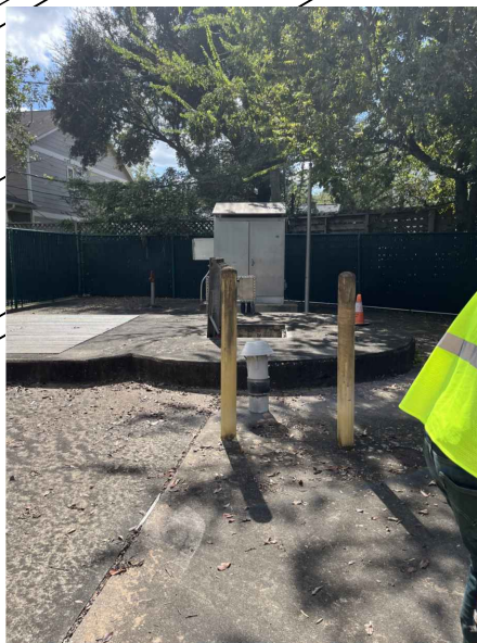
EXISTING LIFT STATION CONTROL PANEL NTS
