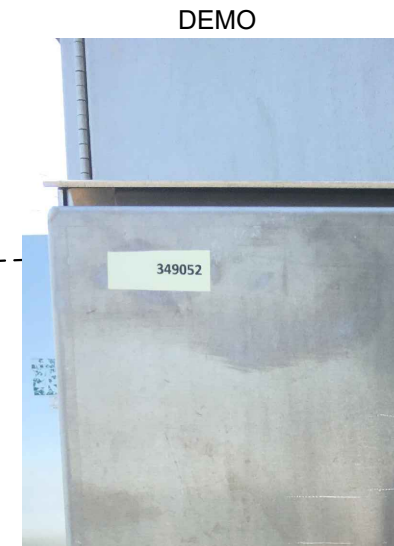
EXISTING LIFT STATION TRANSFER SWITCH
