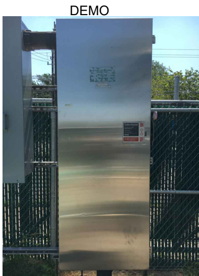
EXISTING LIFT STATION MAIN DISCONNECT
